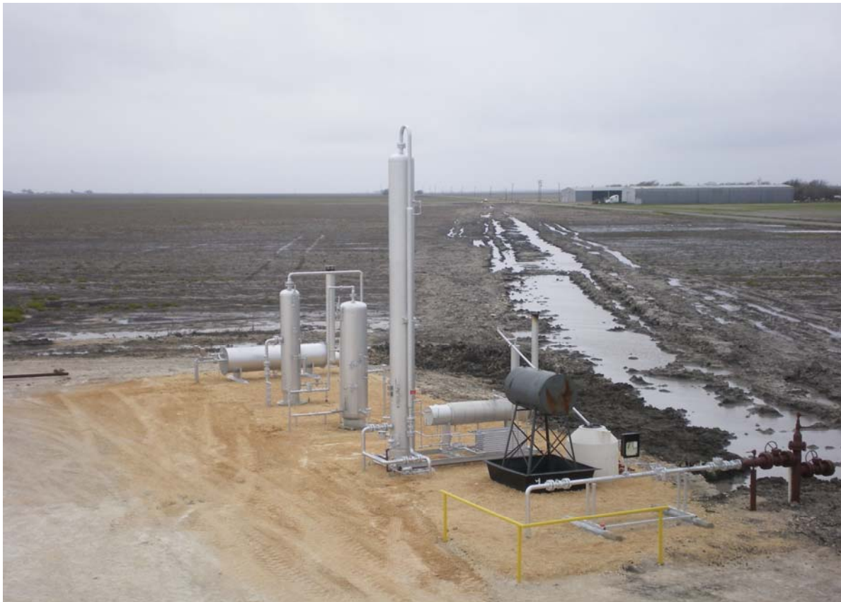
Figure 1 – processing facilities at the Smith #1 well site
